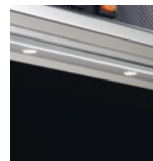
Illuminazione a led Led lighting
